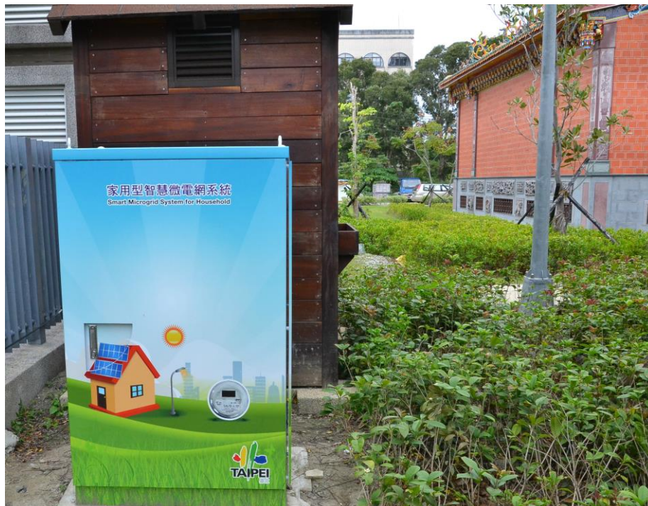
Figure 2: energy storage system (including energy management system).
