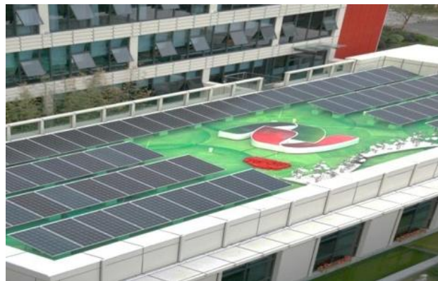
Figure 11 Roof PV project on the SPIC's smart campus
