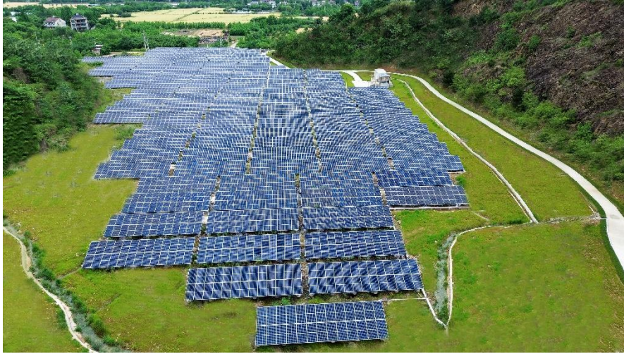
Fig. 4-7 Photovoltaic Power Generation Project in the Abandoned Xinjiang Mine
