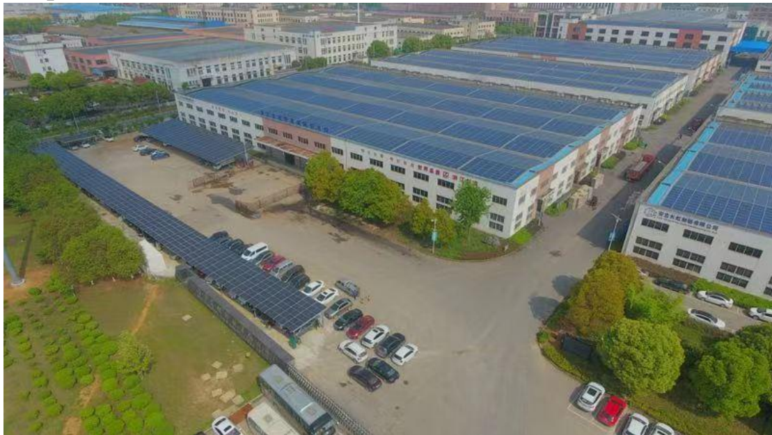
Fig. 12 Huzhou Changhong Generation-grid-load-storage Integration Demonstration Project
