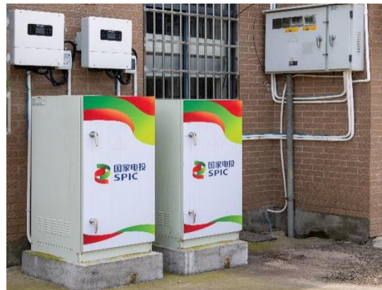
Fig. 4-5 Home Energy Storage Devices
