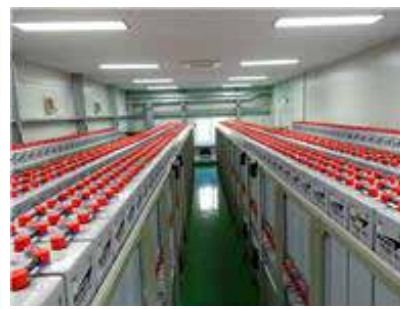
▲ Lead acid battery ESS
