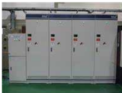
▲ Lithium polymer battery ESS
