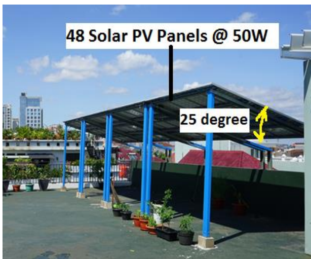
Figure 18: 48 pcs Solar PV Panel @ 50W
