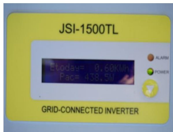
Figure 20: Display of on grid solar inverter
