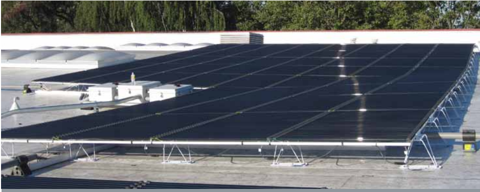
(Clockwise) The historic façade of the Central Maintenance Facility, the power controller for the solar PV array, and the completed installation of the rooftop solar PV array.
