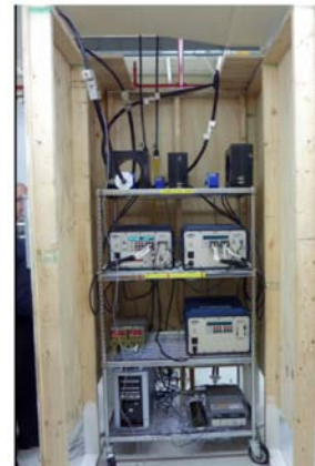
Three Phase 320 Amp Current Source for Electrical Meters
