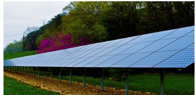
50kW PV Array supply 400-600Vdc, 135A dc
